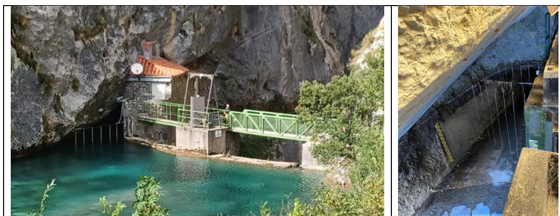
Figure 21. Caín hydroelectric dam and the electric barrier installed to avoid the entrance of fishes in the diversion channel.
