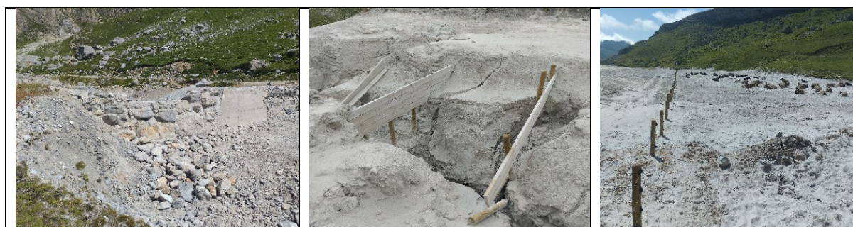
Figure 11. From left to right, containment dike, broken wood sheet piles and livestock exclusion fencing.
