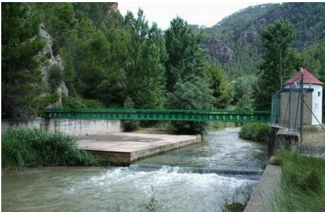
Figure 59. Example of a traditional gauging station installed on the Júcar River.
